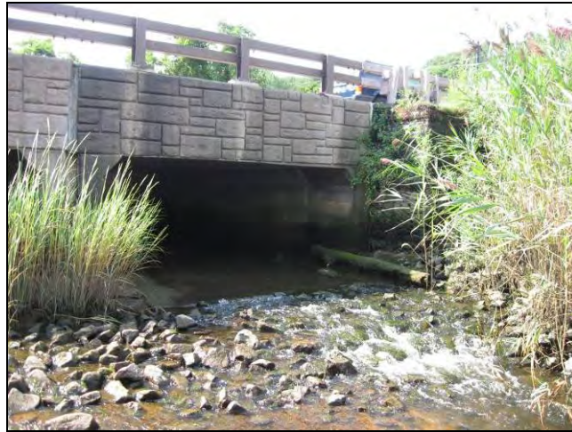
SC-03 is a twin box culvert beneath Route 25A along reach CSB-01.
