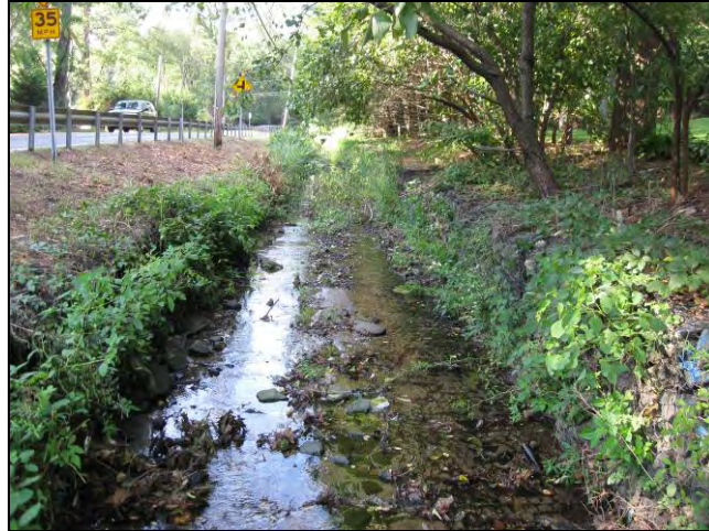
Reach CSB-05(CM-03) consists of a modified stream channel with gabion wall banks.
